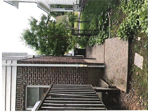
EXISTING SIDE WEST CONCRETE PAVING BEHIND THE MUDROOM ENTRY TO BE REMOVED
